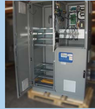
2 x 125Vdc-75A with battery cabinet
